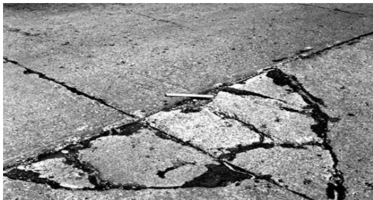
Gambar 2. 7 ( Edge Cracking ) Cacat Tepi Perkerasan
